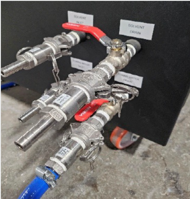
Figure 12 - Process fluid connections
