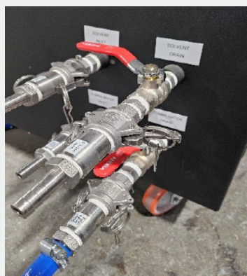
Figure 4 Process fluid connections
